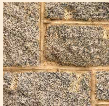
A section of wall on the western wing showing pale coloured scars, evidence of the hammer and tap method used to quarry the granite. Photo, GL
